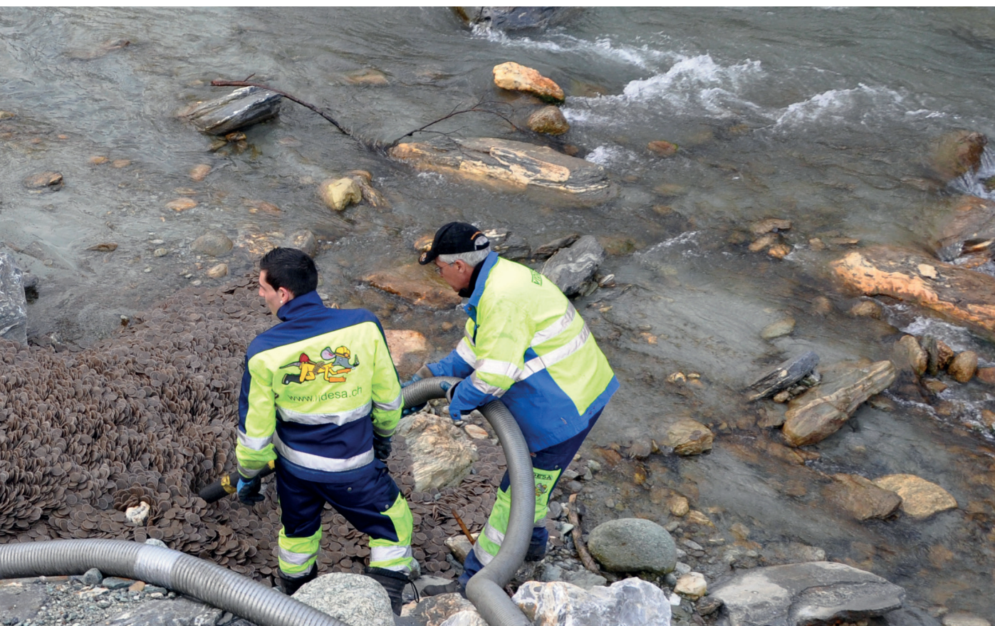
Illustrations | Below | Recovery operation after an important leakage in Evolene, Switzerland in 2012. © Commune Evolene
