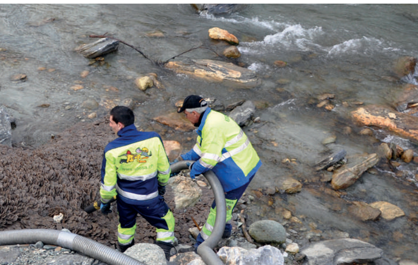
Illustrations | Below | Recovery operation after an important leakage in Evolene, Switzerland in 2012. © Commune Evolene
